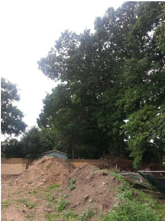
View along line of trees showing protective barrier not in place and debris in RPAS
